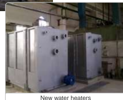
New water heaters
